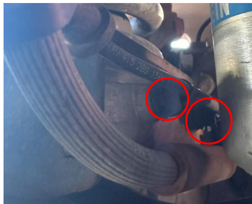
Coil bucket zip ties to be cut
